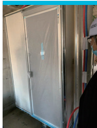
Figure 1.3.1.2-1 Modular bathroom with an RFID tag attached to its roof plate
